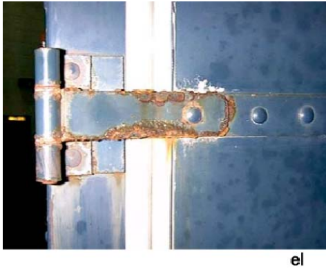
Figure 6-6. Galvanic Corrosion Steel Hinge Bolted To An Aluminum Door
