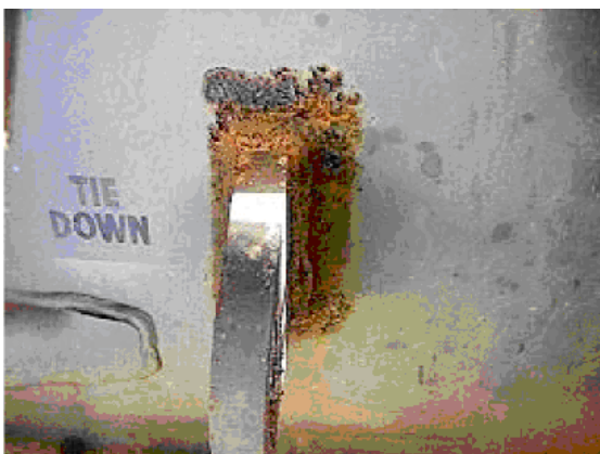
Figure 6-17. Corrosion on Weldments
