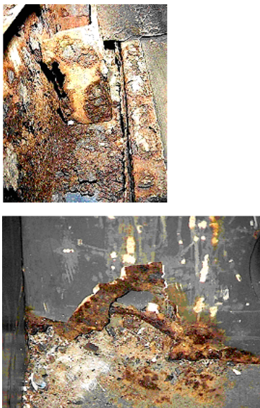
Figure 6-15. Corrosion Resulting from Long-Term Exposure to Sand
