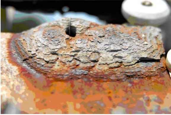
Figure 6-4. Example of Raised Corrosion Product
