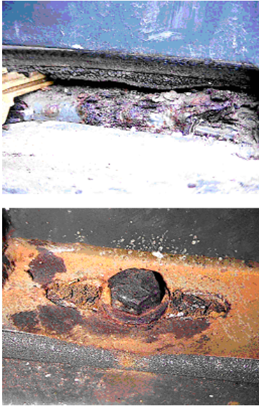
Figure 6-14. Open Cell Foam and Resulting Corrosion
